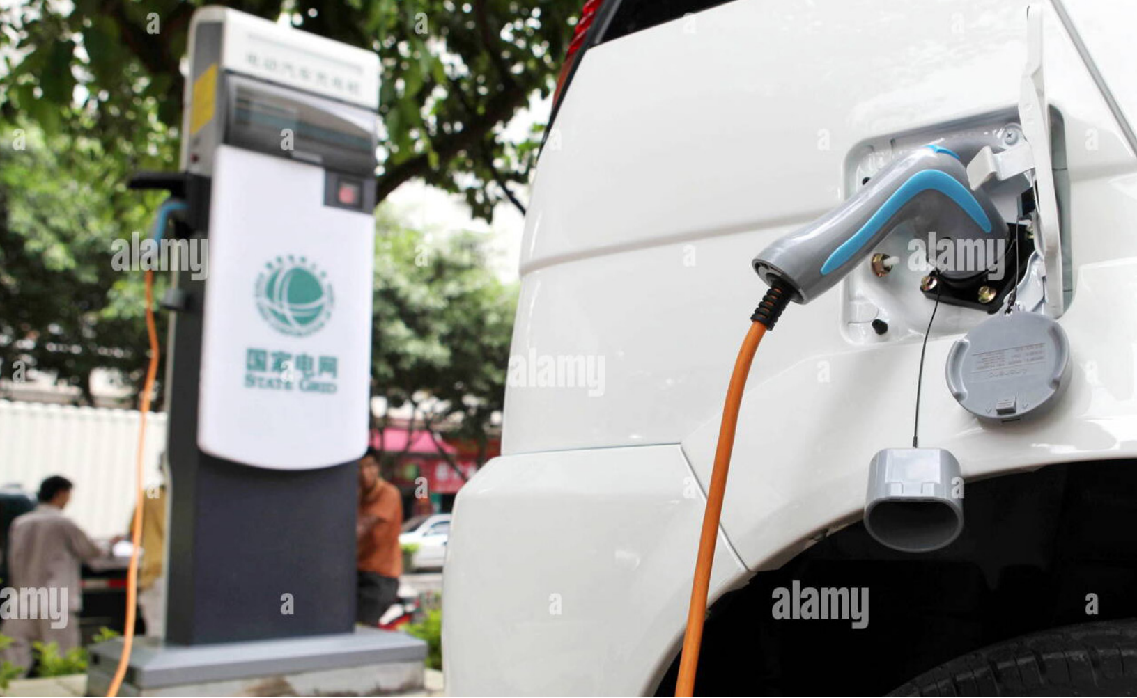
Photo: An electric car is being recharged during the launch ceremony of a charging station of State Grid Corporation of China in Xiamen city, southeast China. Credit: Imaginechina Limited / Alamy Stock Photo
